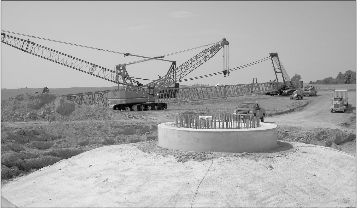
Pictured above, one of the 27 pads for wind turbines, with the crane used in background.
