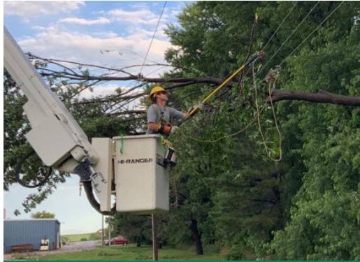
Pictured grounding the line is Eric Becker. Grounds are applied to assure the line is dead (off) and safe to work on while making necessary repairs.
